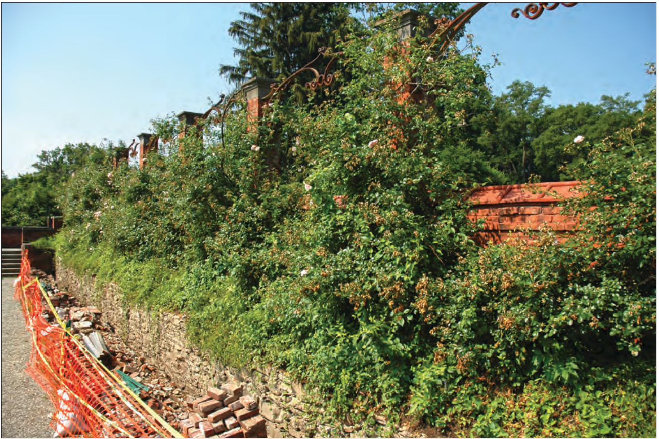
2.33. View south of repairs to the retaining wall on the upper west end of the rose garden. Climbing roses in the bed above the wall extend up to the wire scrolls between brick pillars, which also frame the east edge of the lower perennial garden (OCLP 2008).
