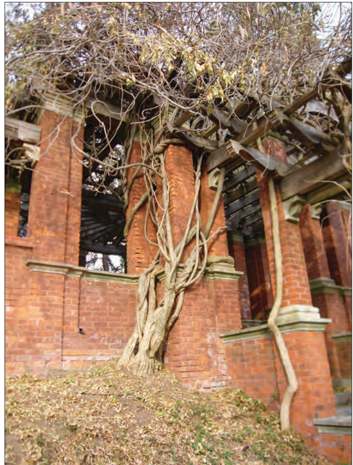
Figure 2.26. View northeast of the north pergola and mature vines. A weep hole in the wall at left allows water to drain from the interior of the pergola (OCLP 2008).
