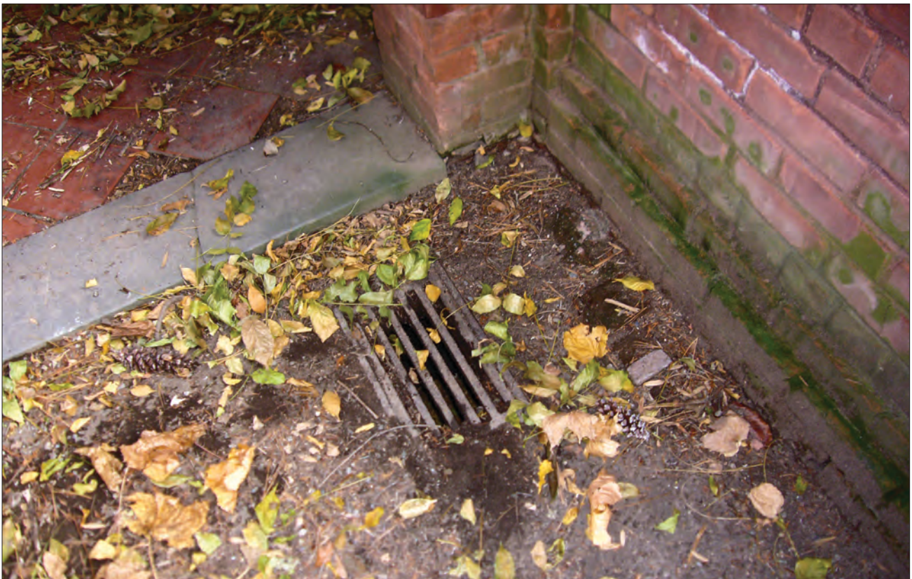
Figure 2.25. Close-up of a drain in the north pergola, a detail specified on the original construction drawings by James Greenleaf (OCLP 2008).
