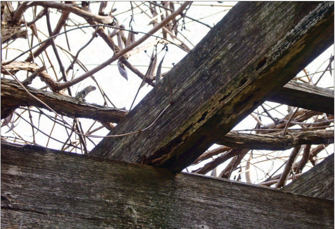
Figure 2.24. Close-up view of the south stair pergola with rot in one of the beams (OCLP 2008).
