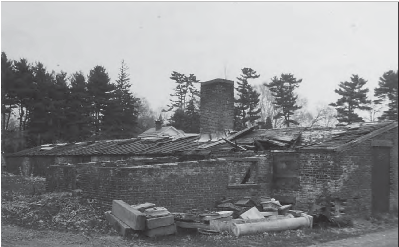
Figure 1.87. View looking northeast showing the damaged Potting Shed with stockpiled elements including columns and bluestone steps, circa 1970s (VAMA, no. 71592).
