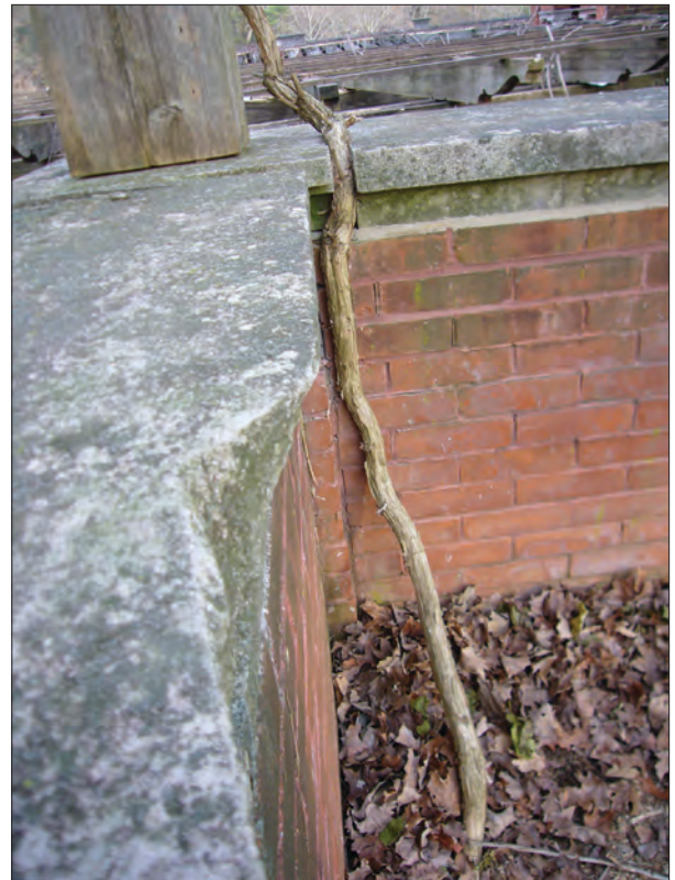
Figure 2.42. Close-up of a trumpet vine by the south stair pergola. The vine is growing between two cap stones, forcing them apart (OCLP 2008).
