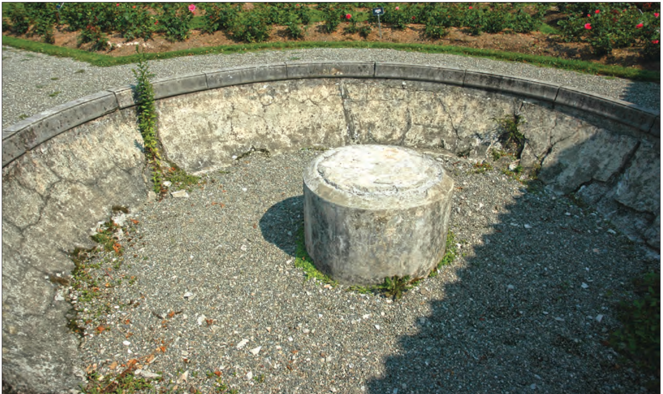
Figure 2.52. The shell of the Orpheus fountain in the lower rose garden is cracked and in need of repair. The Orpheus fountain and pedestal which were placed at the center of the fountain in 1925 were removed in 2005 due to overall spalling and erosion and are currently undergoing conservation treatment (OCLP 2008).
