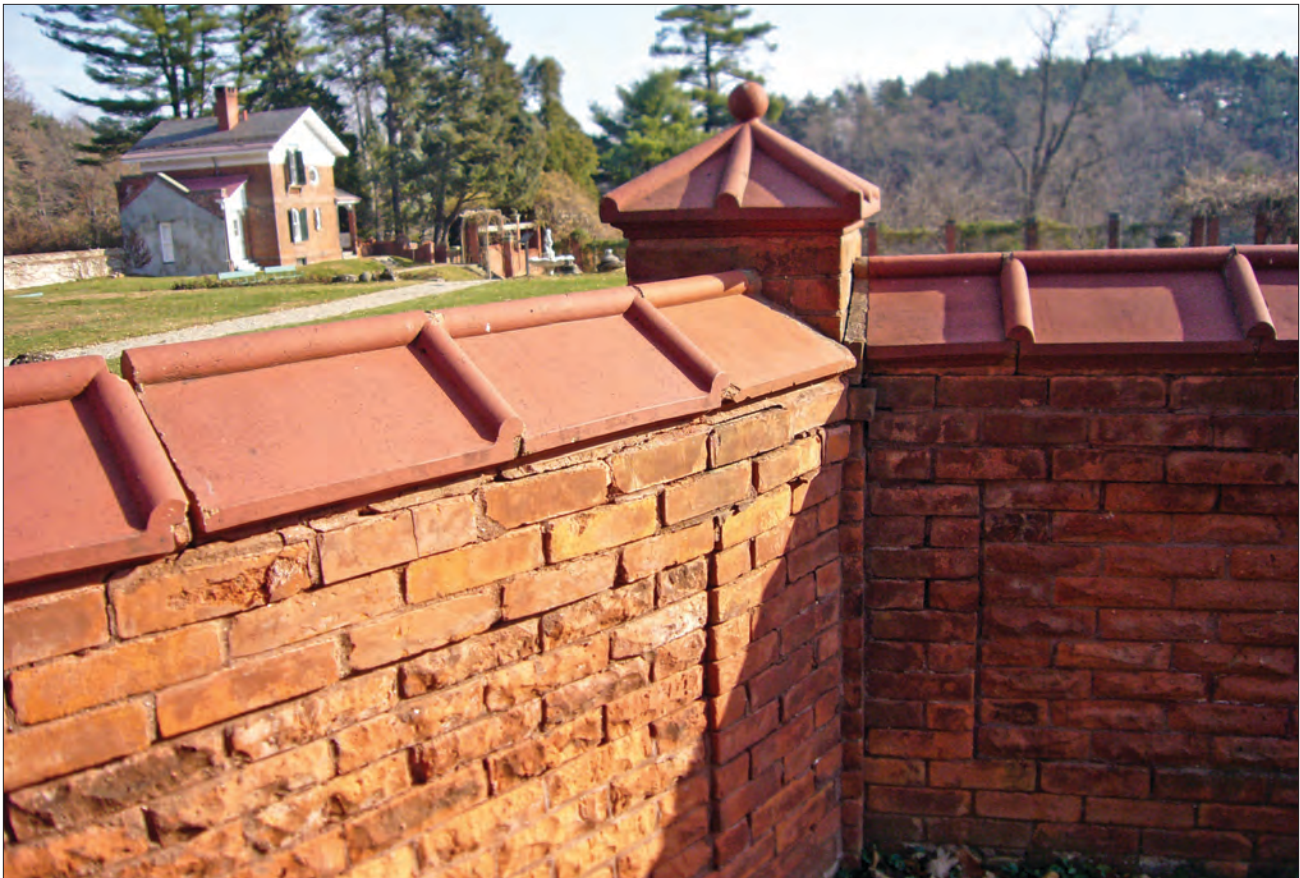
Figure 2.20. View east of a remaining red clay finial on top of the garden wall. Most of the finials have been broken off by vandals. The capstones are intact and the wall section is in good condition with only minor cracks (OCLP 2008).
