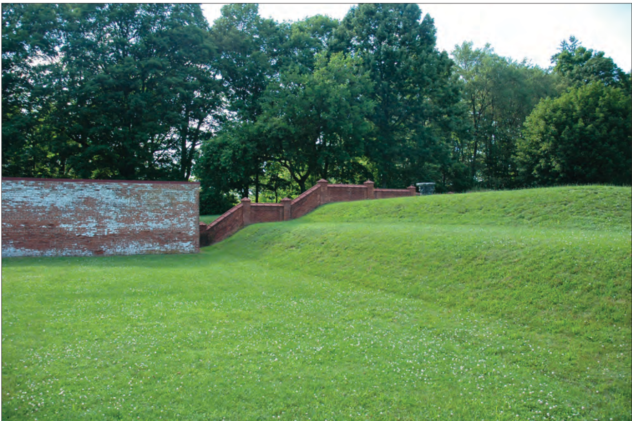
Figure 2.4. View west of the greenhouse terraces from the site of the former Rose House (OCLP 2008).
