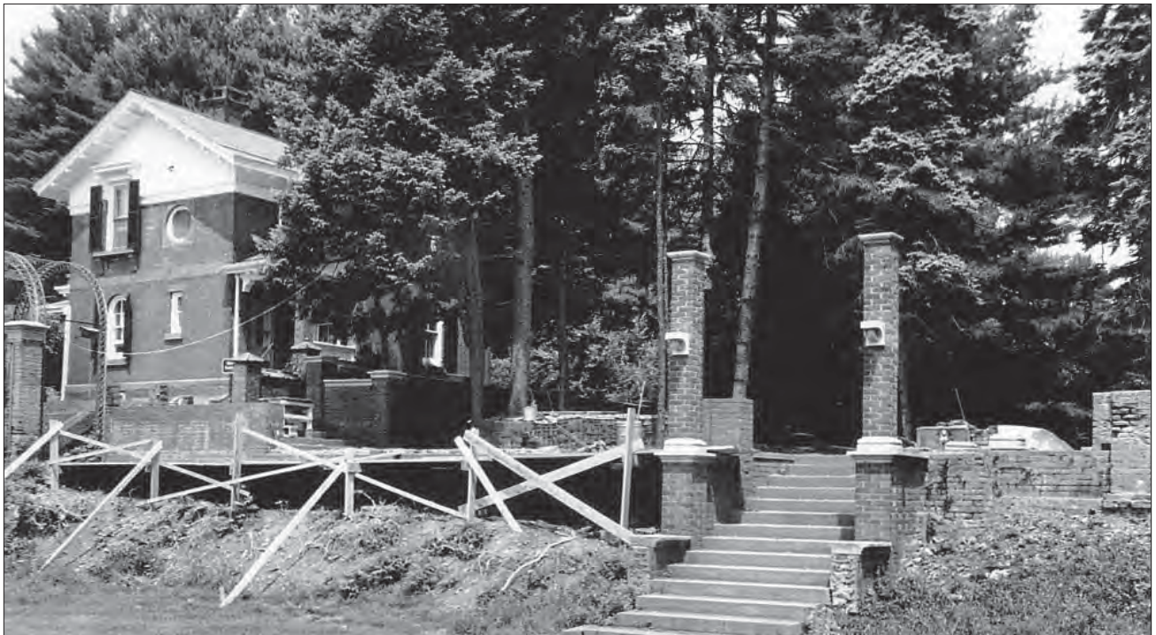
Figure 1.89. View looking north showing the north pergola under rehabilitation, circa 1970s (VAMA, no. 5012, F. W. Vanderbilt Garden Association Collection).
