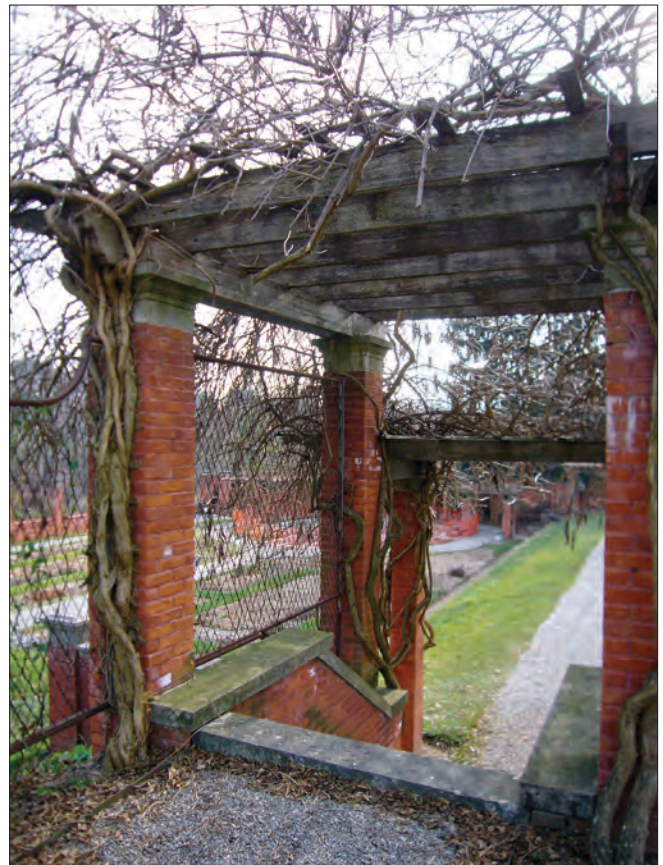
Figure 2.23. View southeast of the central stair pergola. Rot is present in several of the wooden beams above the walkway, which support the weight of the vines (OCLP 2008).
