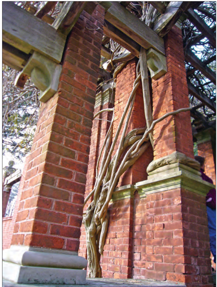
Figure 2.16. Close up view of the vines encircling the brick piers of the north pergola (OCLP 2008).
