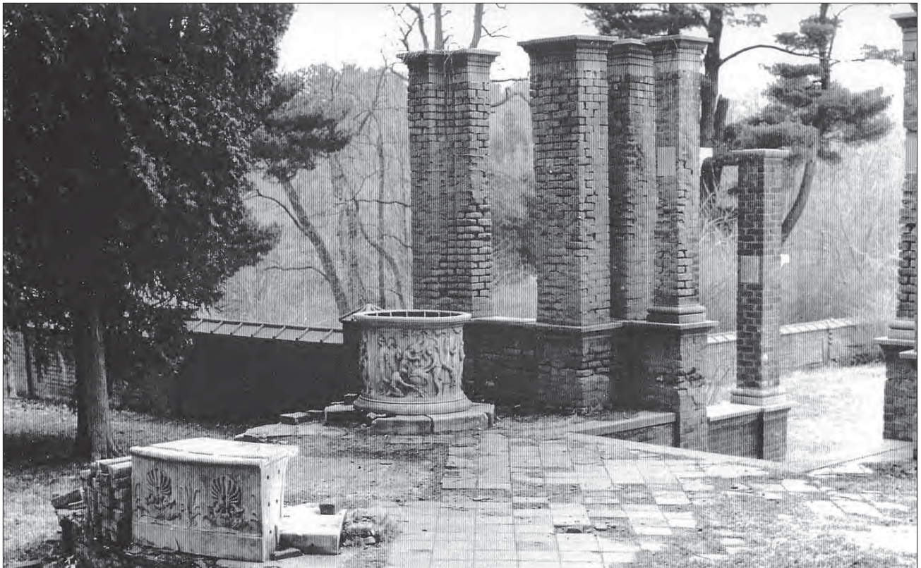
Figure 1.88. View looking southeast showing the remnants of the north pergola, circa 1970s (VAMA,5006, F. W. Vanderbilt Garden Association Collection).
