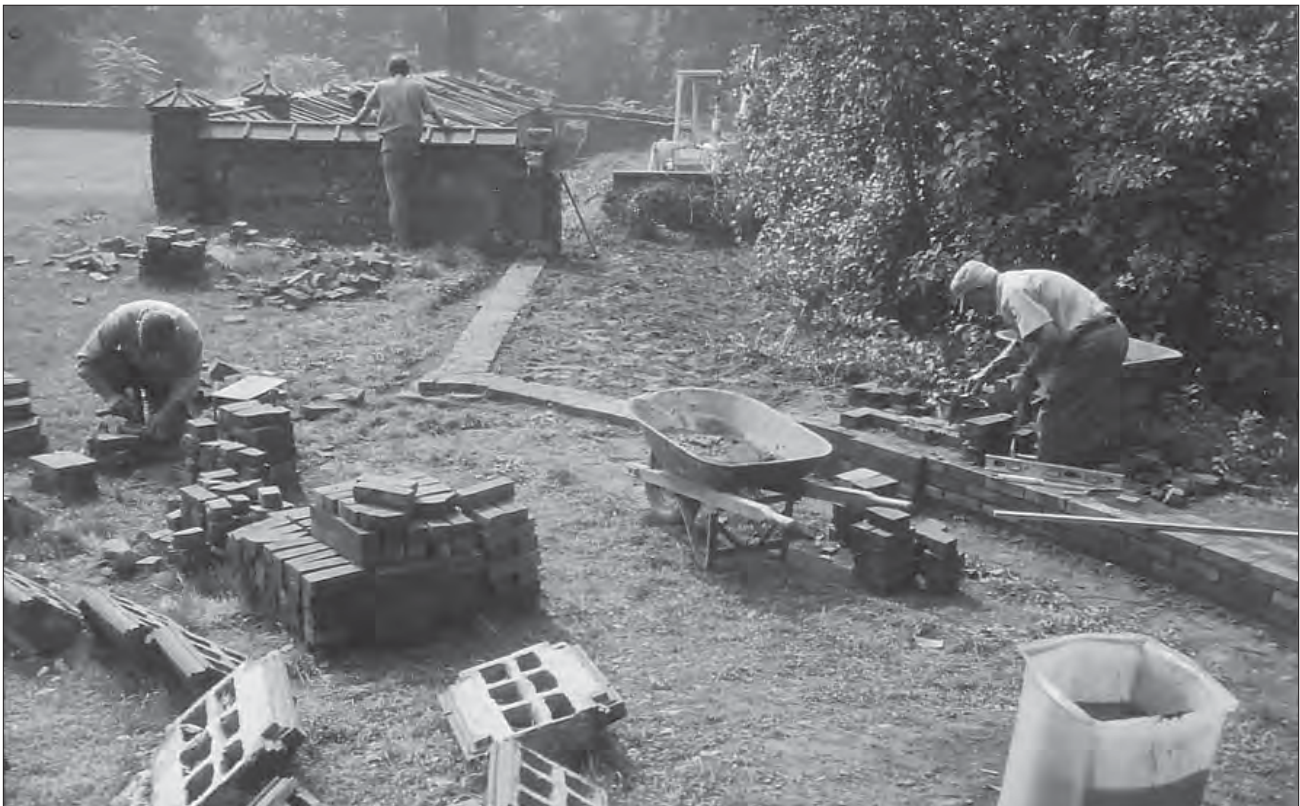
Figure 1.91. View looking south showing repairs being made to the garden wall, circa 1970s (VAMA, no. 1025, F. W. Vanderbilt Garden Association Collection).
