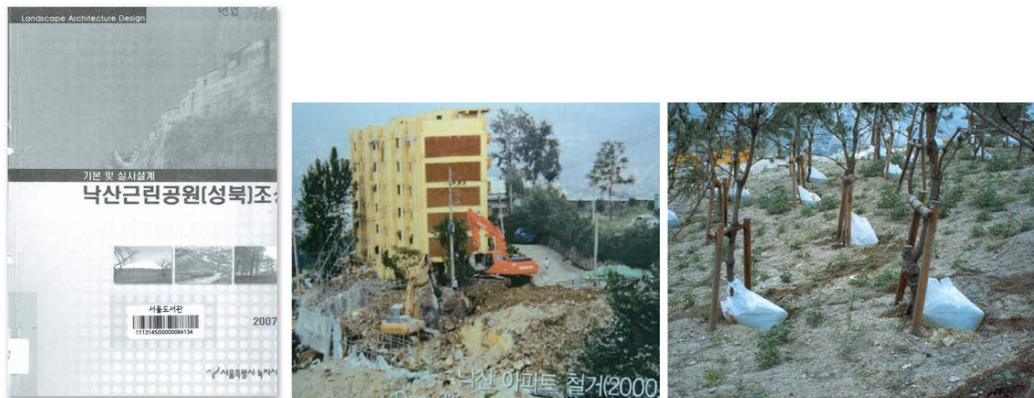
41 | Demolition of Naksan citizen apartments and reforestation based on the Naksan Restoration Plan (@ Seoul Metropolitan Government)
