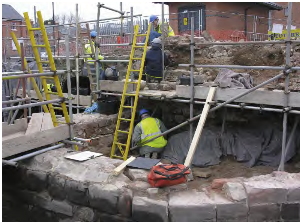
Fig 99 Conservation work and archaeological recording in progress on the bridge fabric, looking east
