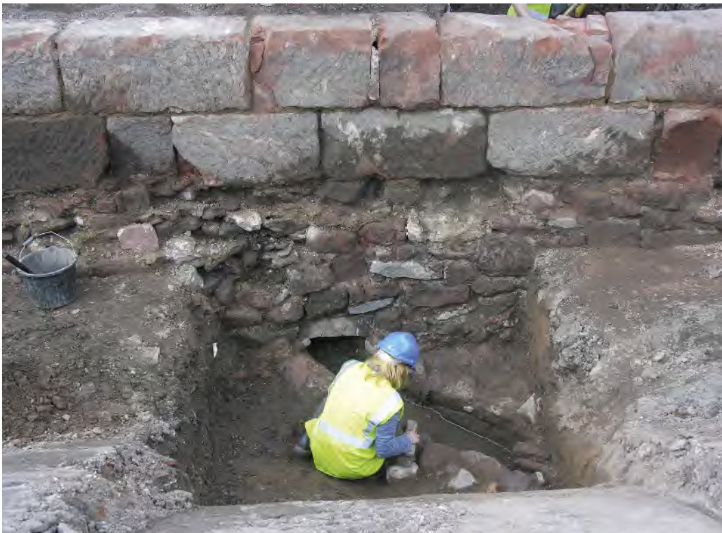
Fig 60 The stone-lined culvert at the base of the barge quay and masonry abutment (S9) under excavation, looking west
