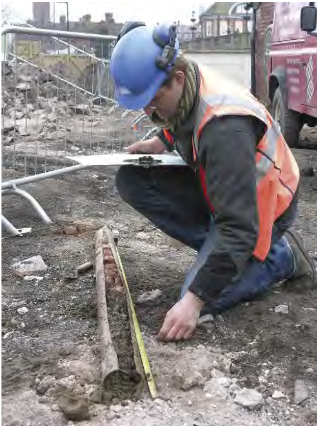
Fig 11 Logging borehole samples on site, with one length of a windowless core sample extracted by the MC300 drilling rig
