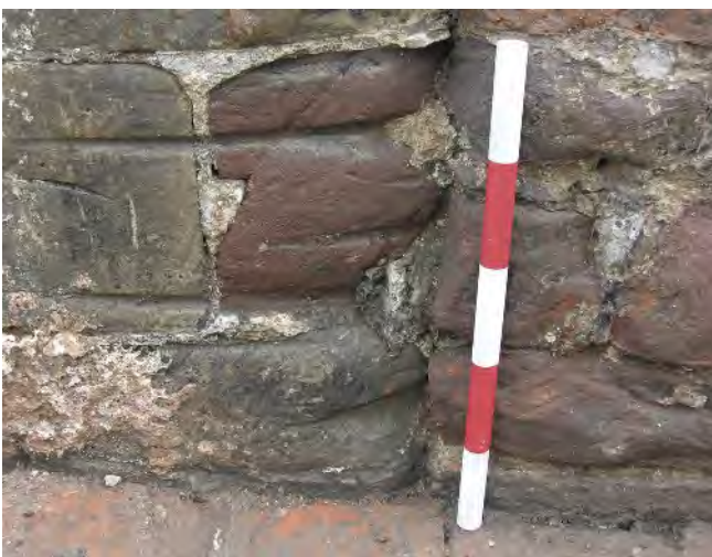
Fig 49 Rubbing marks on the north-west corner of the west bastion (B11), looking south (0.5m scale)
