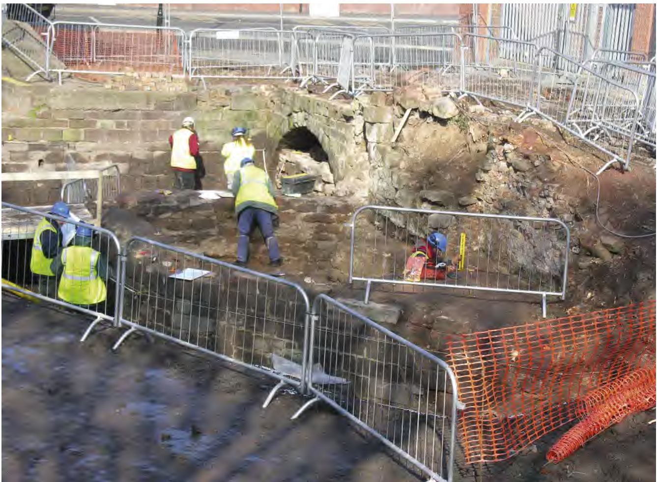
Fig 3 The masonry structures within the area to the west of the bridge arch being recorded during March 2006, looking north
