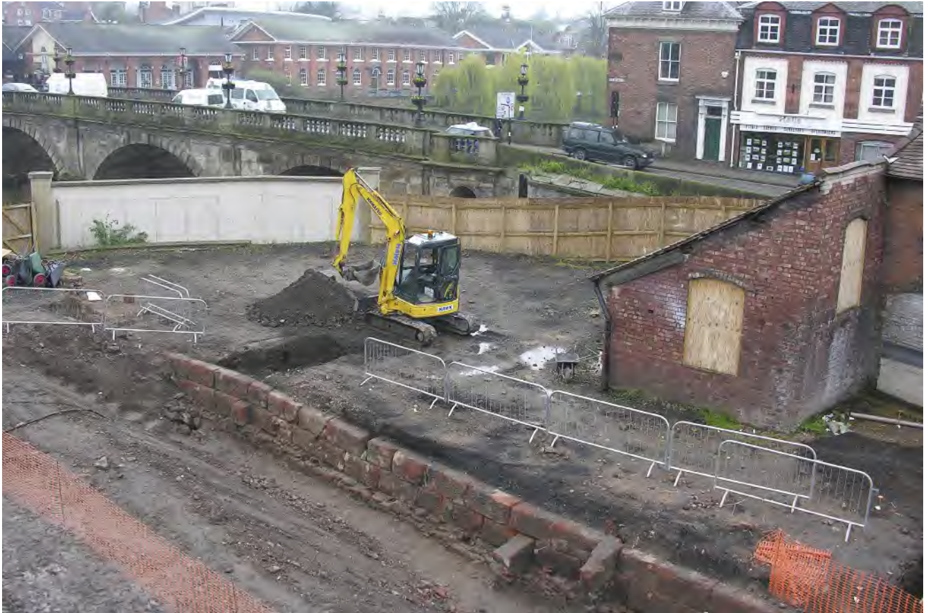
Fig 57 The external (eastern) face of the barge quay and masonry abutment (S9) being uncovered, showing the southernmost of the two trenches excavated on the west side of the wall; to the rear is the new Welsh Bridge, looking south-west
