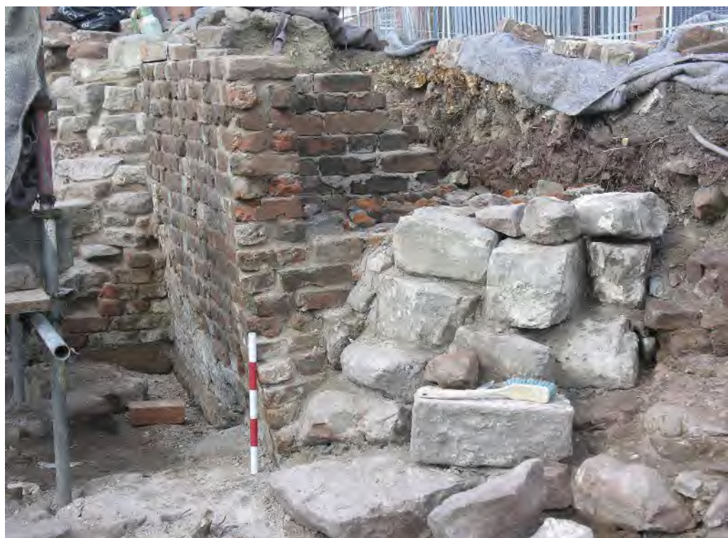
Fig 100 Brickwork [46] along the southern side of the bridge fabric after rebuilding and repair, looking north (0.5m scale)
