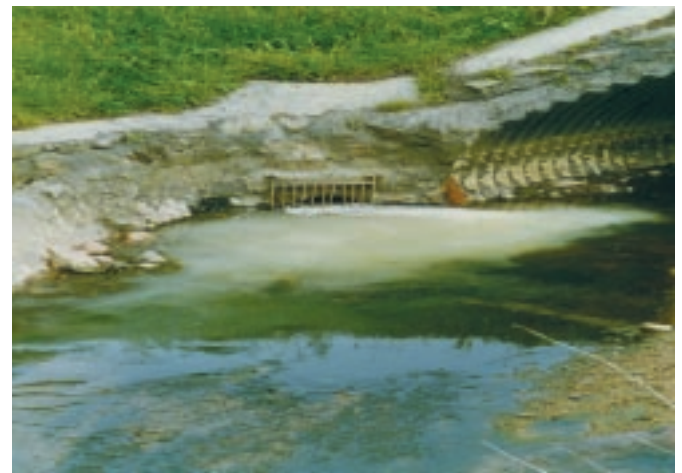
Figure 1. Potentially damaging direct discharge into an urban stream.
